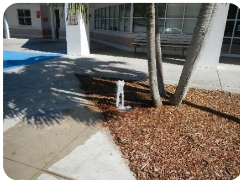
Broken sprinkler heads are a common problem encountered during irrigation evaluations at schools.
